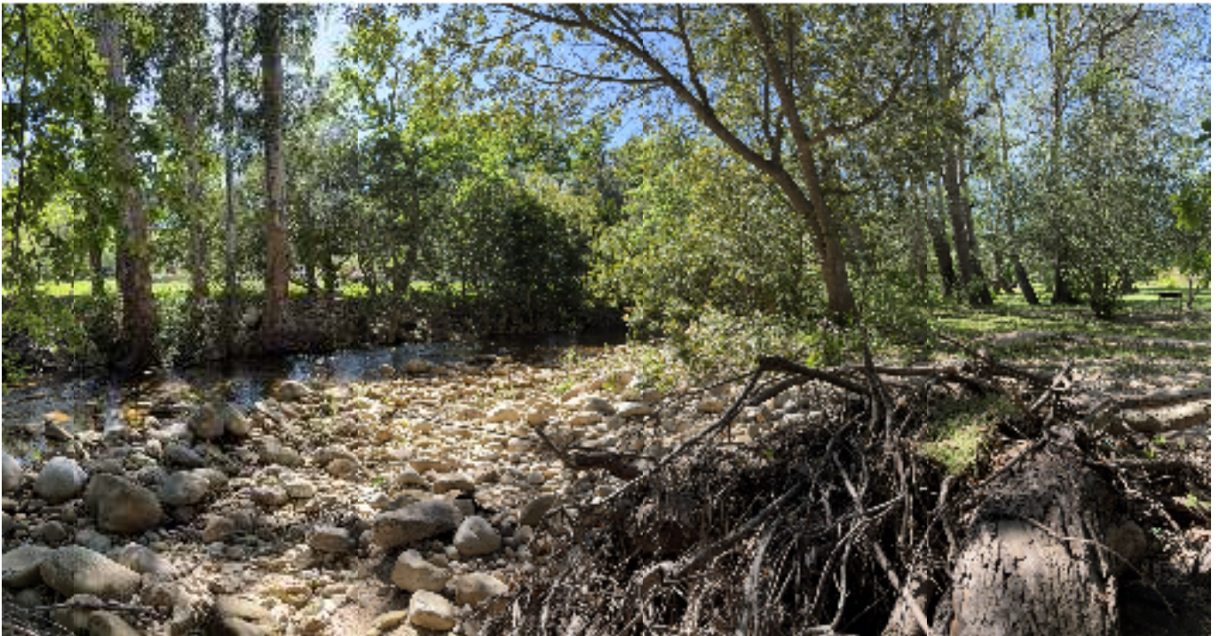
Bank erosion on opposite bank, downstream of House Richter due to 2023 flooding
