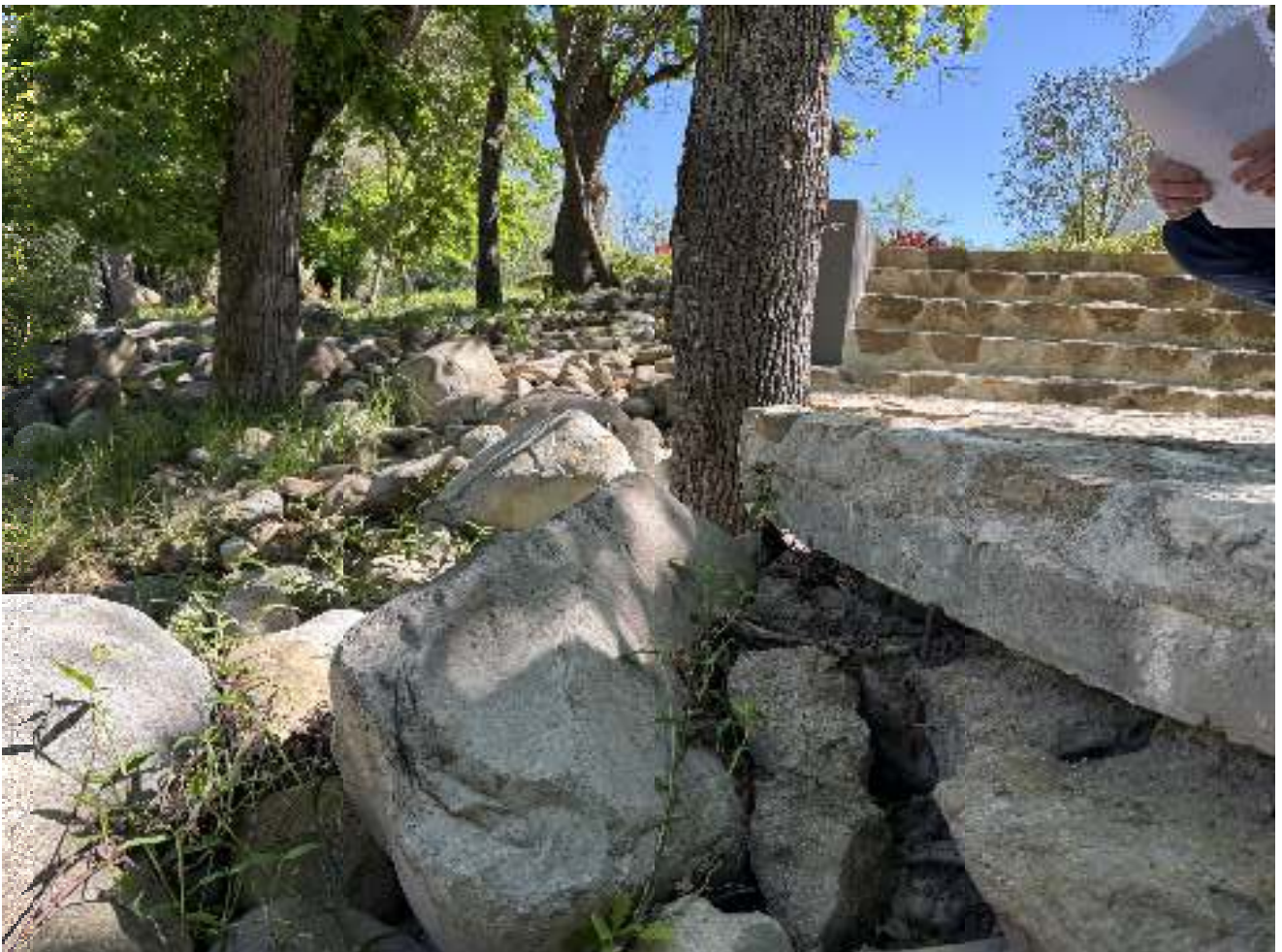
Braai area structure undercut by 2023 flood
